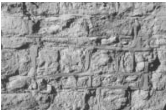
Overhard cement based repointing will damage the stone as this prevents moisture evaporating through it.
