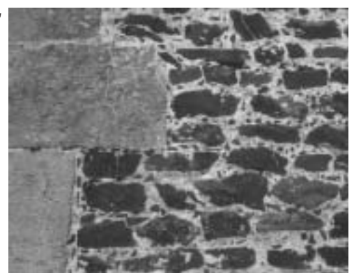
An ironstone wall with sandstone (churt) quoins and galletting (stone chips) in the mortar joints.
