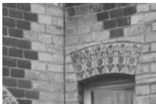
The pointing on this building is soft and just back off the arris (edge) of the brick - it does not need repointing just because the mortar joint is soft and can be raked out by hand. The joint is doing its job allowing moisture to evaporate from the masonry.
